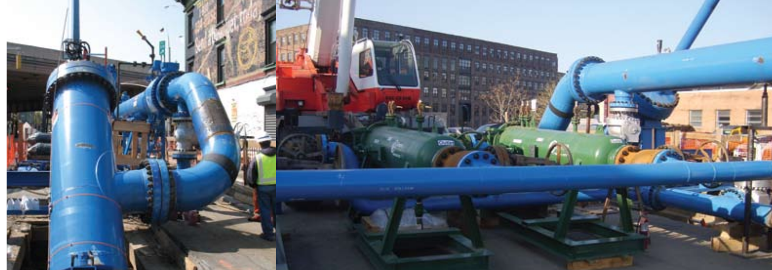
Launch (L) and receive (R) sites were located in a High Consequence Area surrounded by busy auto traffic and densely populated residential and business districts.
